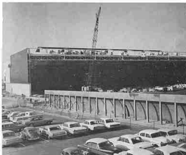
PSA'S NEW MAIN OFFICE-HANGAR facility nears completion as massive steel trusses are secured and roofing of five-plane hangar gets under way. Tieback sections weight 16 tons and will support the 400 ft. wide hangar plus the three-story administration building which will give PSA 3 1/2 times its present space.
