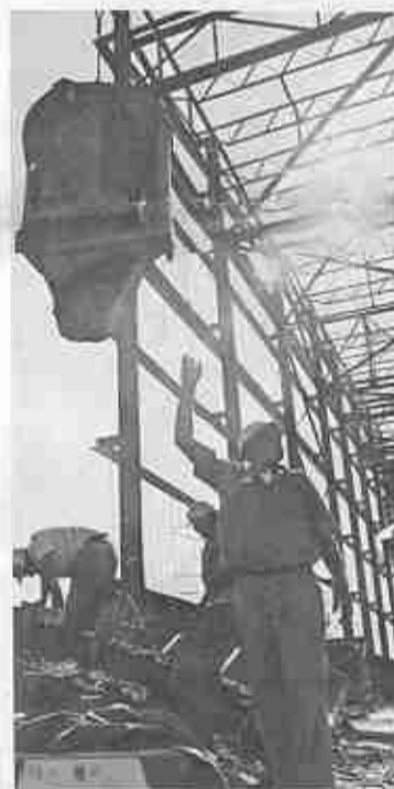
CEMENT is poured into molds which form sections of the blast wall being erected adjacent to the new facility. Blast walls are necessary as a back-up to start jet engines, and will line both sides of the maintenance area.
