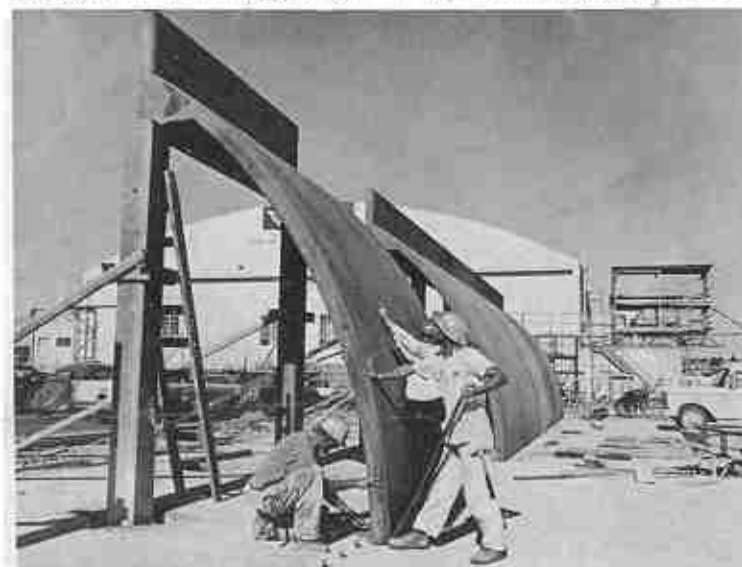
SECOND BLAST WALL is inspected by Paul Sweeney, center, general superintendent for building contractors Haas & Haynie, as workers Bill Suttles, left, and Russ Groening secure cement section of precast.
